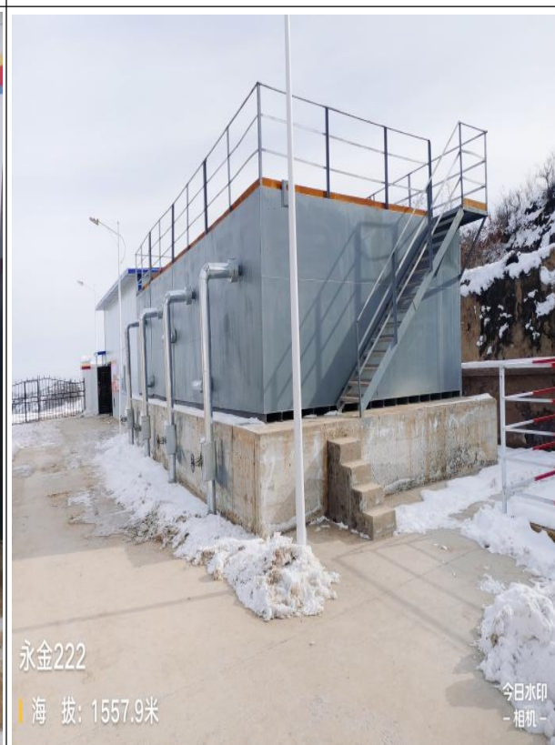
50m 3 污水沉降罐
